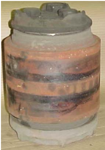
BEARING BEFORE RECONDITIONING
